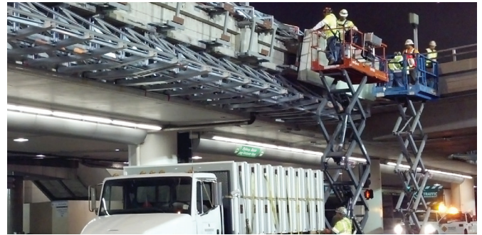
Early-morning installation of the light band and art-deco light poles in front of TBIT. Work on the Curbside Appeal Project is carefully coordinated and phased in order to limit impacts on motorists and pedestrians.
